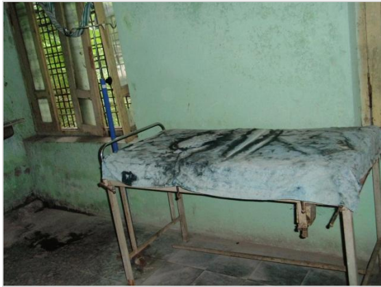
Labor room with broken windows
