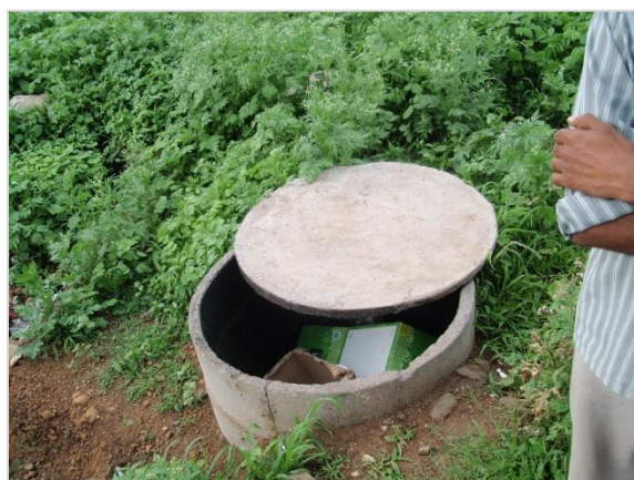
Waste disposal in backyard of a PHC
