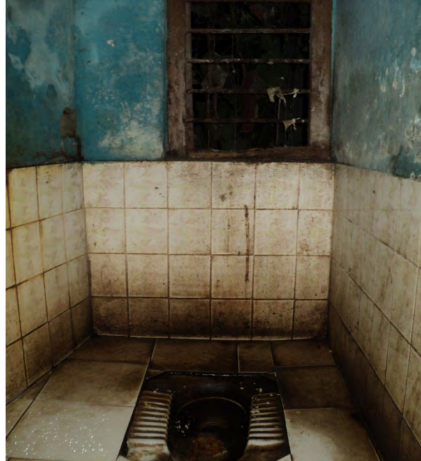
(Condition of Maternity ward toilet of SDH,
