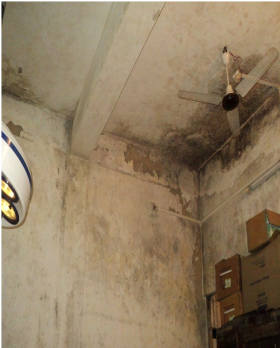
(DH: Laproscopic OT room with Plaster peeling off)
