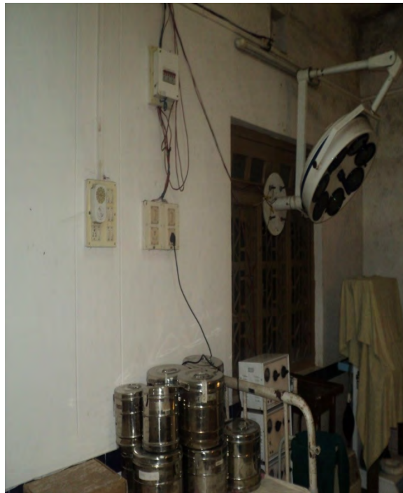
(DH: Exposed Wiring just above the OT table)
