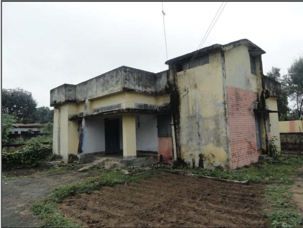
Figure 1: Dilapidated Condition of Residences at RH Amarpur (05th Nov 2012)
